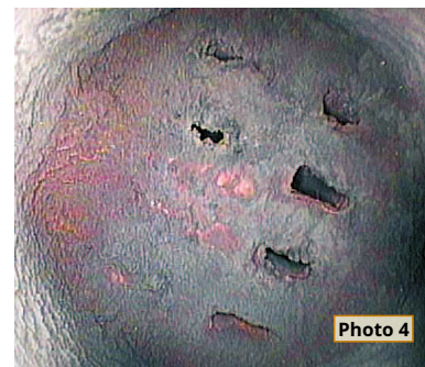
Photo 4 shows an oxide plugged water hose manifold. This is not copper corrosion, but rather what the evidence shows. The observed oxide deposits primarily result from the redeposition of \text{Cu}(\text{OH})_2 copper hydroxide which accumulated as \text{Cu}_2\text{O} and \text{CuO} .
